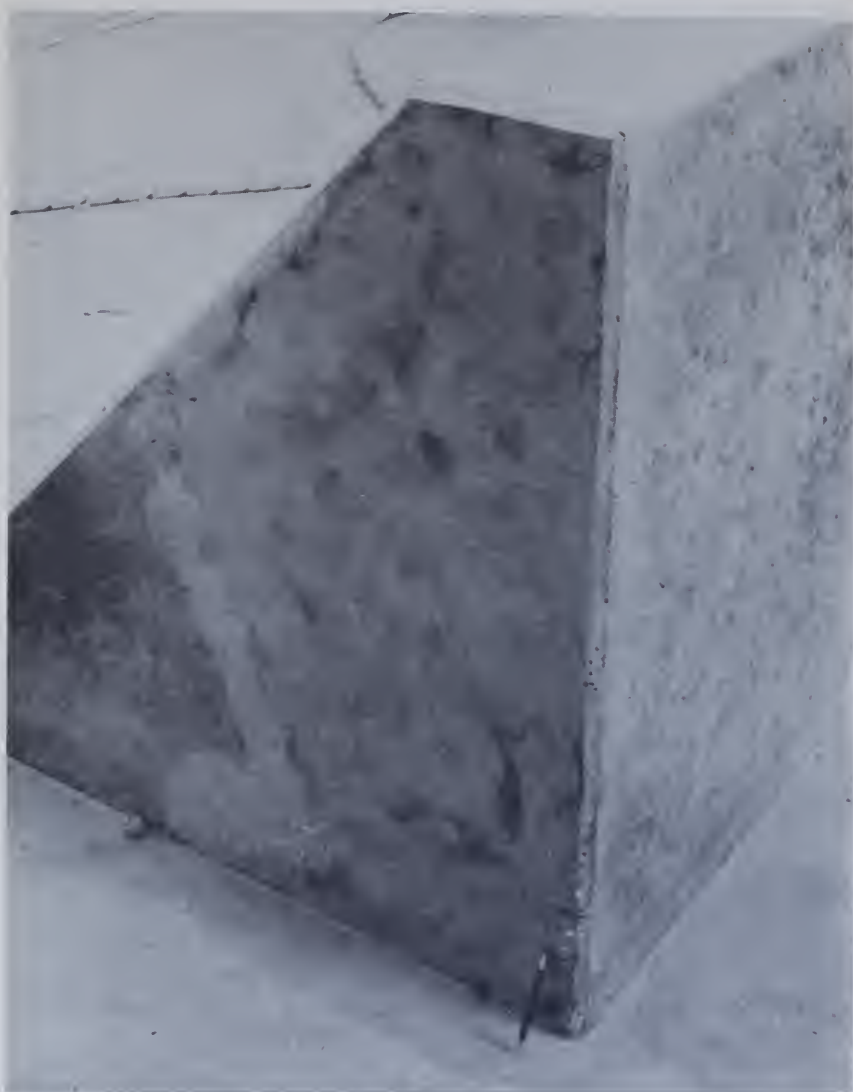
Figure 186.—A damaged dentate in overflow weir stilling basin at Yellowtail Afterbay Dam restored to its original condition with epoxy-bonded epoxy mortar. The concrete color of epoxy mortar was obtained by grinding after completion of curing. P459-D-68915.
